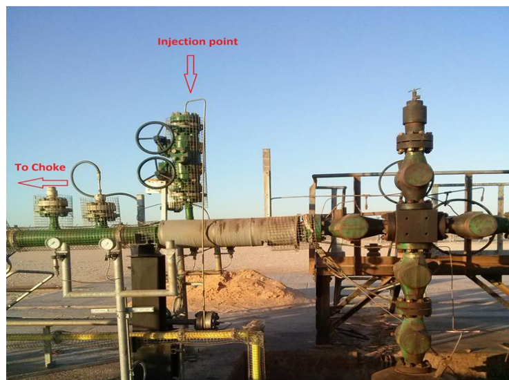
Figure 16. The permanent surface up choke dilution water pumping system (1/2" injection line).
